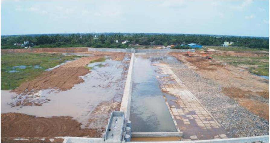
Check dam constructed across Gadilam river in Vilangalpattu village in Cuddalore district at a cost of Rs. 12.50 crore from DMFT Fund
